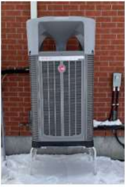
Rheem Heat Pump, July 2023.
