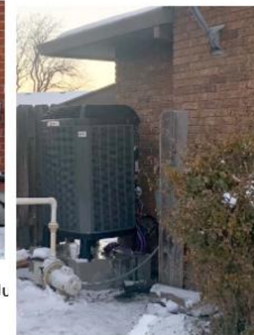
A Trane Heat Pump, July 2023.
