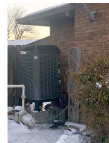
A Trane Heat Pump, July 2023.
