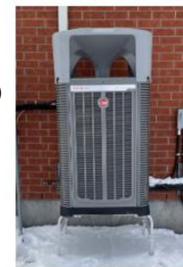
Rheem Heat Pump, July 2023.
