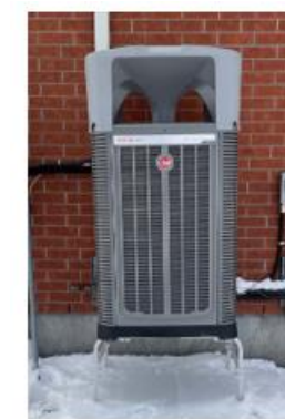
Rheem Heat Pump, July 2023.
