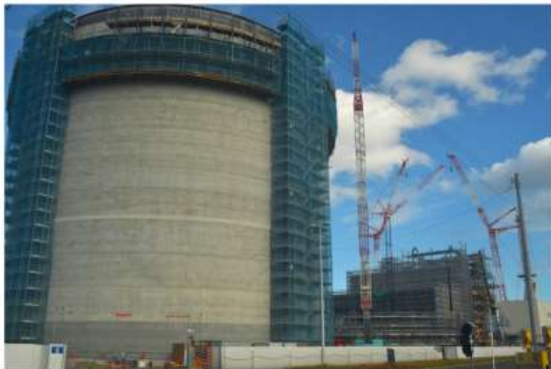
A plant under construction in Japan will soon join the many burning wood pellets to generate electricity.
