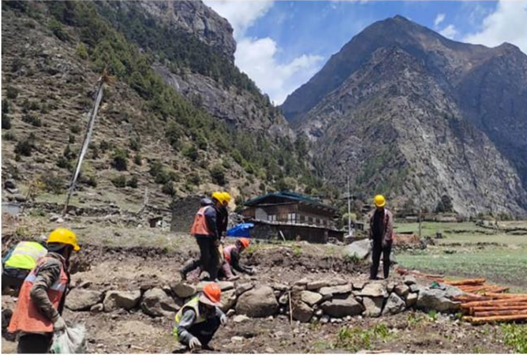
June 12, 2024 Shangsa village in Lunana is set to benefit from clean and reliable energy by August this year. [The work is underway to install a solar system for the 10 households of the village.
