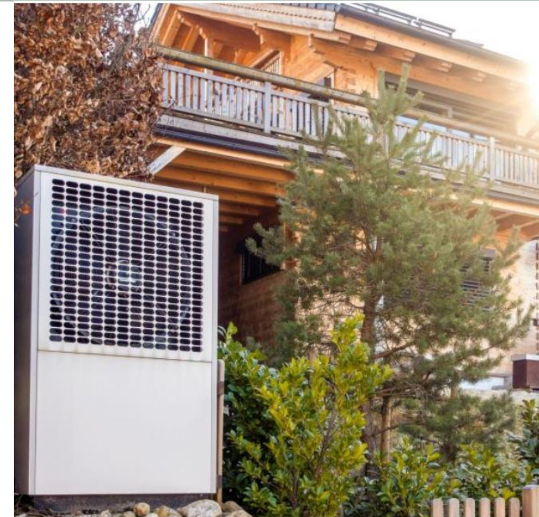
A modern heat pump in front of a residential building in Bavaria, Germany.
